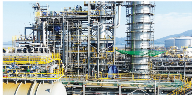
SNG Pipe Insulation
