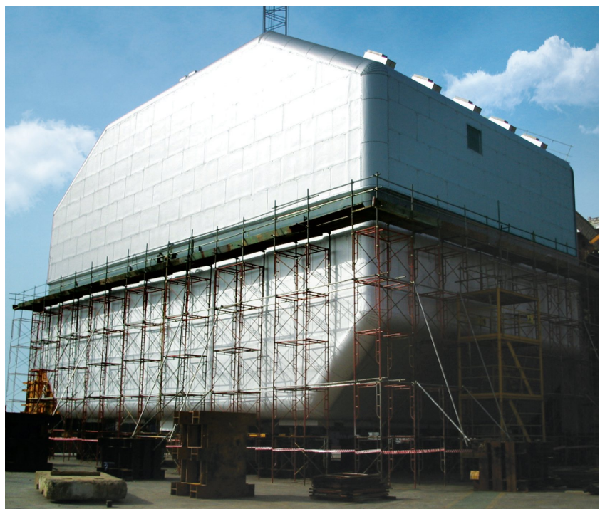
Prismatic Type LPG Cargo Tank Insulation
